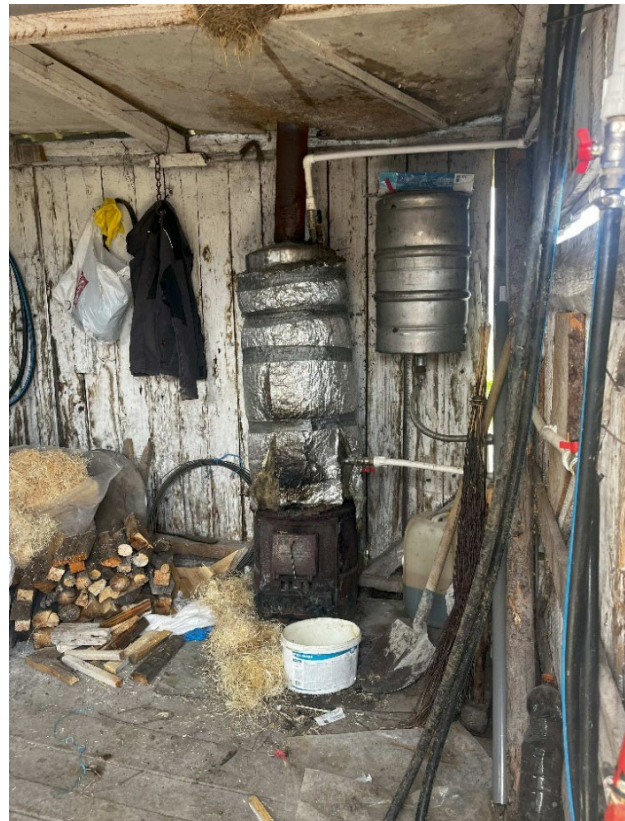
Figure 10: A converted wood-fuelled bathing furnace to produce hot water.
